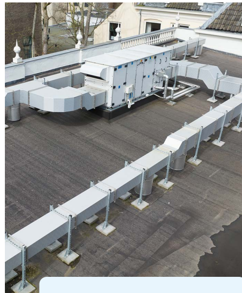
Dakopstelling LBK, R-vent
