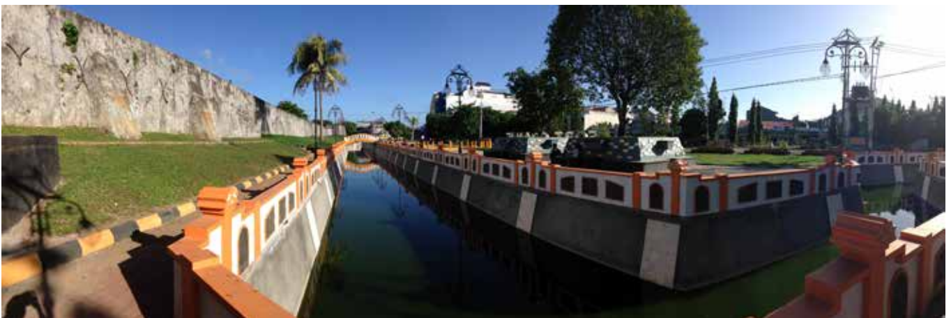
The Dutch Fort Oranje in Ternate (Indonesia), recently restored (photo: Maulana Ibrahim)
